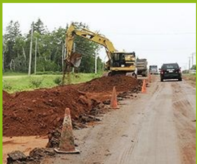
Many infested areas arise as a result of road construction
